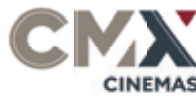
Workmen were on the jobsite Tuesday where the CMX Cinébstro movie theater is under construction at Coastland Center mall.
